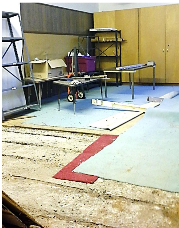
Demolition of the unsafe floor in the former preschool room is underway.
