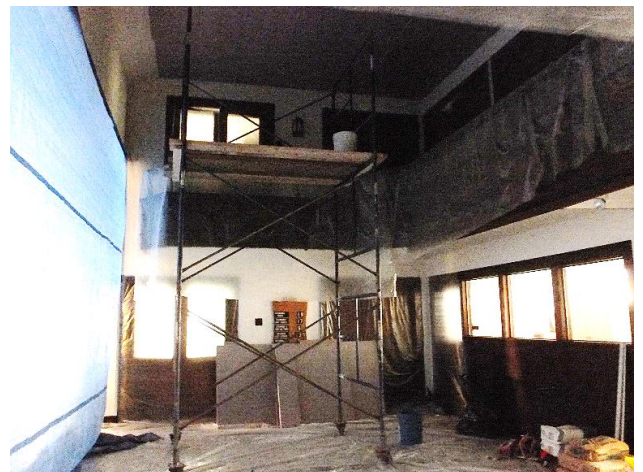
Scaffolding was set up and the repairs started in the overflow area.
