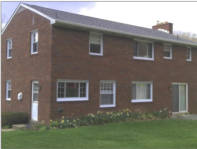
3. In this photo, all of the windows in the back of the house have been replaced. Do you see the difference between the old and new windows?
