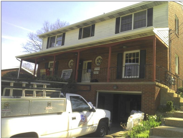
1. New windows have been installed on the first floor. The old windows are still in place on the second floor.
